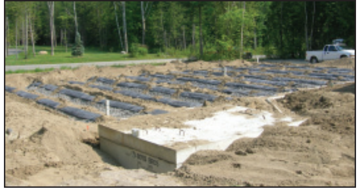
Septic tank and leaching bed.
